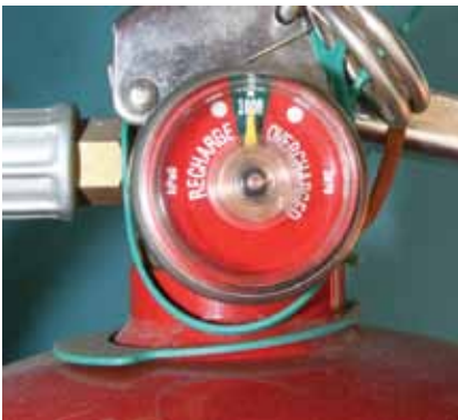
Extinguishers need to be replaced if not charged
